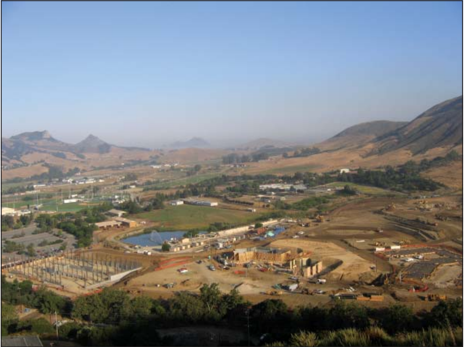
Student Housing Project, Cal Poly, San Luis Obispo, CA — “The best way to have a good idea is to have lots of ideas . . . .”
